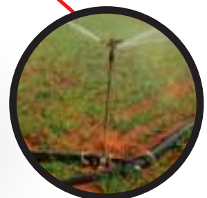
Irrigation & Dust Suppression System
